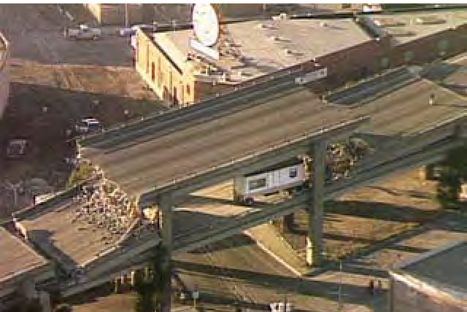
Loma Prieta, CA 1989
